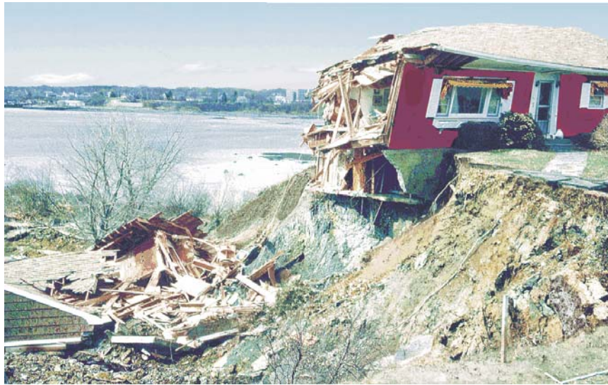
Landslide damage in Rockland, Maine in 1996. See Berry et al., (1996) and MGS (1997) for more information on the 1996 landslide. MGS file photo.
