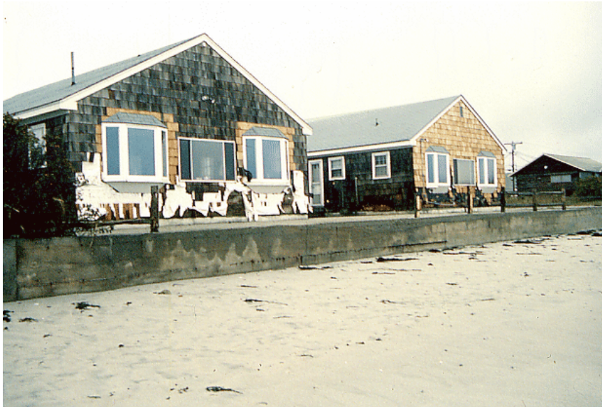
Higgins Beach after the 1991 Perfect Storm. Coastal flooding overtopped the seawall and waves damaged several homes. Photo by S. M. Dickson, 11/01/91.
