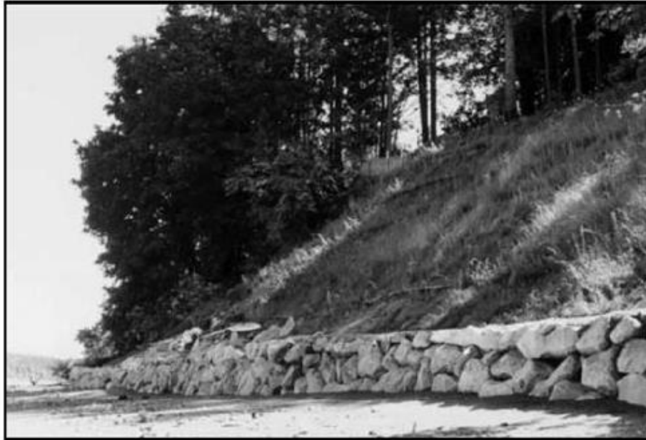
Figure 2. View from the beach. The lift layers can be seen. The slope is approximately 1H:1V, compared to its original near-vertical pre-construction state. The bluff is 30+ feet tall (the rock bulkhead is 5-6 feet high).
