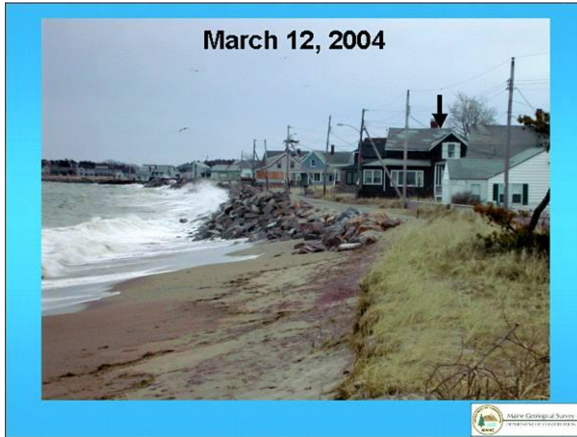
Photograph from March 12, 2004 after a northeast storm. Note full erosion of fill sand at the end of the seawall and seawall settlement.
