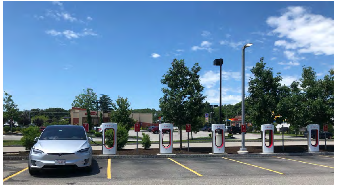
A bank of EV Superchargers in Seabrook, NH. Photo: Tom Morgan.
