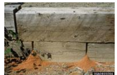
Retaining wall with tell-tale piles of frass.
