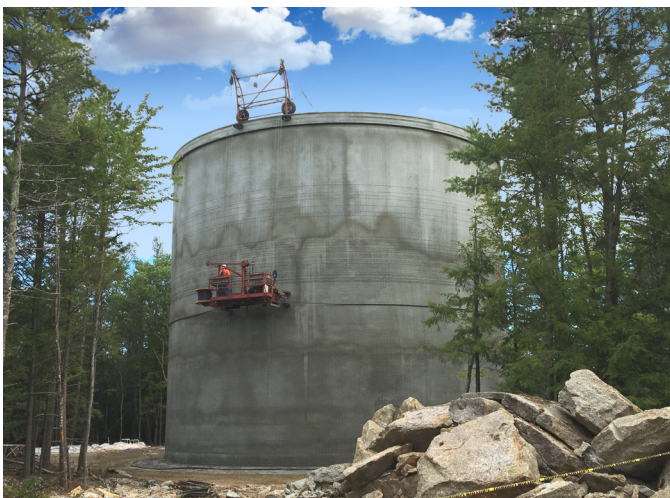
Kennebunk, Kennebunkport & Wells Water District's new 1.5 million-gallon water storage tank in Arundel was completed in 2021 with DWSRF funds. (Photo: McKenzie Parker)
