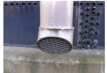
Tank overflow with screening prevents entry from animals
